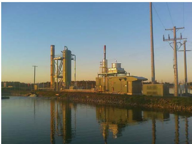
Biogas extraction at Shepparton
